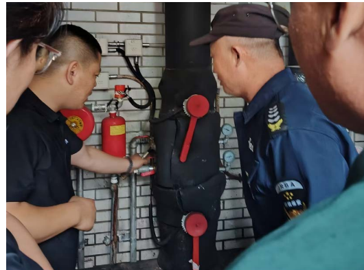
Training for fire control room personnel
