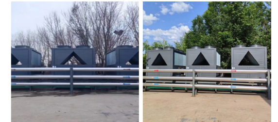
Modern Dairy Saihan Farm air heating equipment
