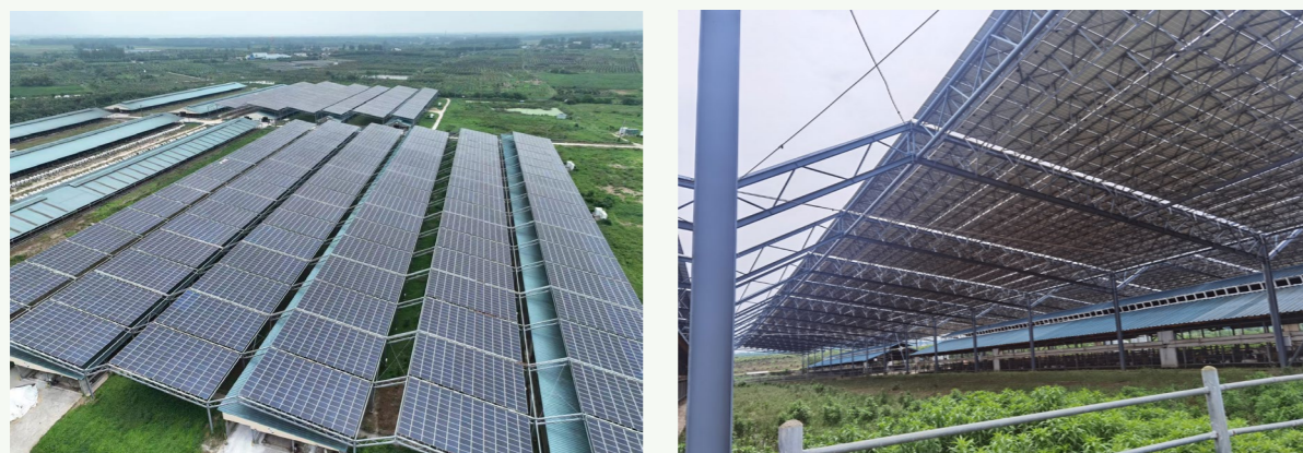
Modern Dairy's Hefei Farm Photovoltaic Power Station
